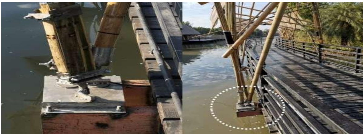
Fig. 7. Actual construction experiment where the pre-fabricated connectors are installed in the locations as they are designed.
