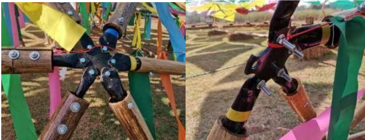
Fig. 13. Images show the real application when bamboo culms are installed with head nozzles, and formed with star plate to make truss frame structure.
